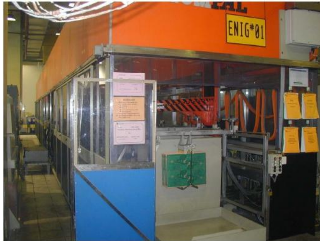
Automated ENIG Plating Line (PAL)
